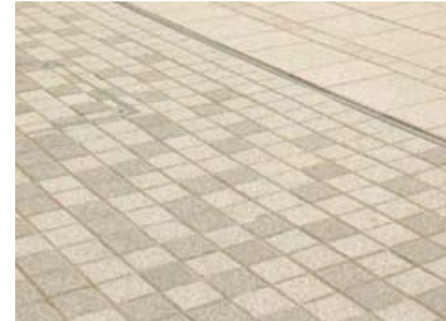
Natural Sandstone setts in New Court
